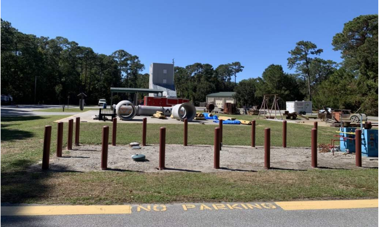
View of extrication pad at left, underground propane tanks in foreground. Project site near white trailer in background.
