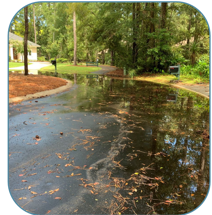
Blocked pipe causes ponding
