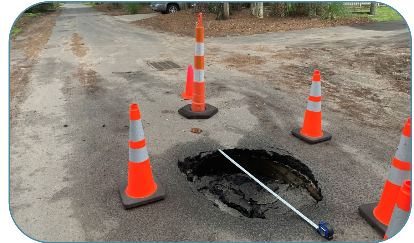
Pipe joint failure causing sinkhole in roadway
