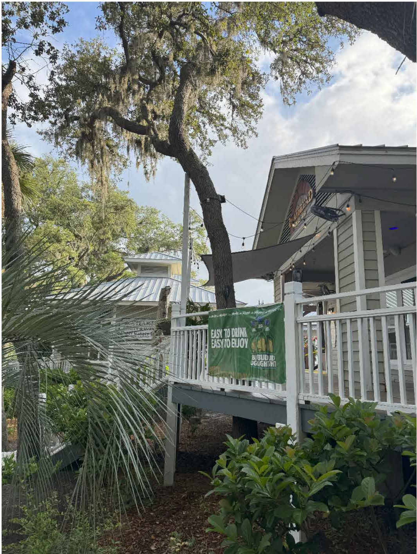
5: 14" LIVE OAK GROWING THROUGH DECK TO BE REMOVED
