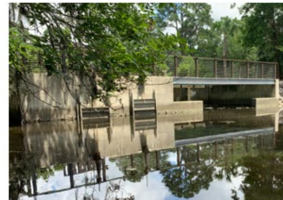
Pump Station Chambers
