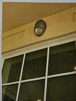
4. LIGHTING FIXTURE – EGRESS LIGHTING
