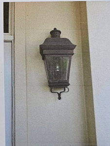
4. LIGHTING FIXTURE – WALL LIGHTS
