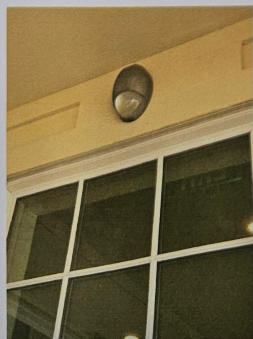
5. LIGHTING FIXTURE – EGRESS LIGHTING
