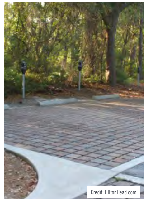
Pervious parking areas, like the system picture above at Islanders Beach Park, allow rain water to percolate into the ground. This helps to re-charge ground water aquifers and minimize run-off.
