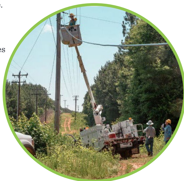
In early 2015, fiber Internet infrastructure was installed on Hilton Head Island, providing residents with high-speed Internet access. Data shows that the average download speeds in the Town (157 MBPS) are currently higher than the statewide and national average, while average upload speeds (30 MBPS) are lower than the statewide and national average. Credit: New York Times
