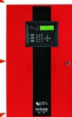
FIRE ALARM CONTROL PANEL (FACP)
