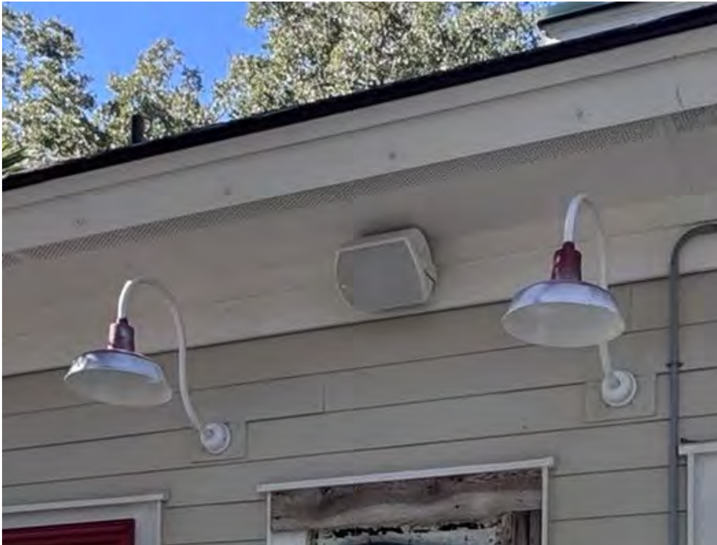
EXISTING GOOSENECK LIGHTS
